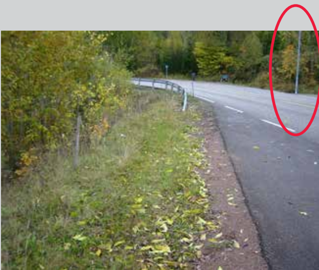
Picture 21 - Problem : lamp post in hazard zone
